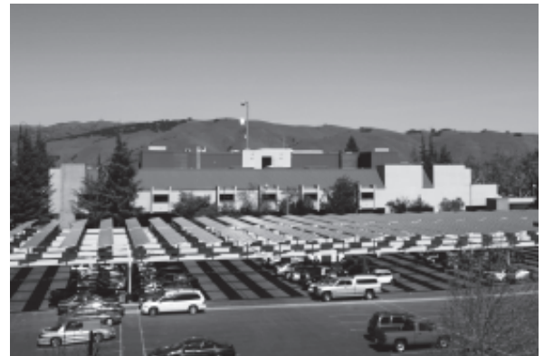
The solar array at the Fremont Hall of Justice
